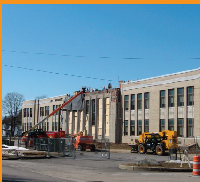
Work continues on the facade of Stamford Central School over the last several weeks. Photo courtesy Ann DuBois
